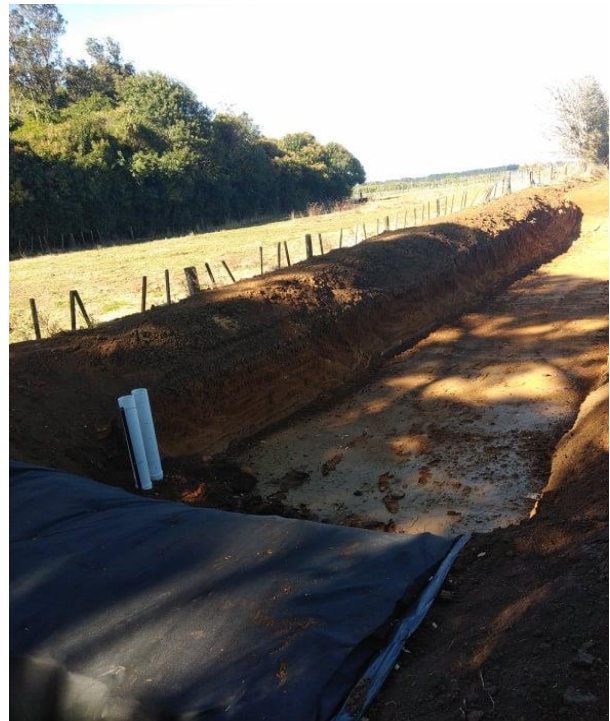
Figure 6. A completed 0.5% SRP. The important elements being volume, snorkels, and a protected level emergency spillway.
